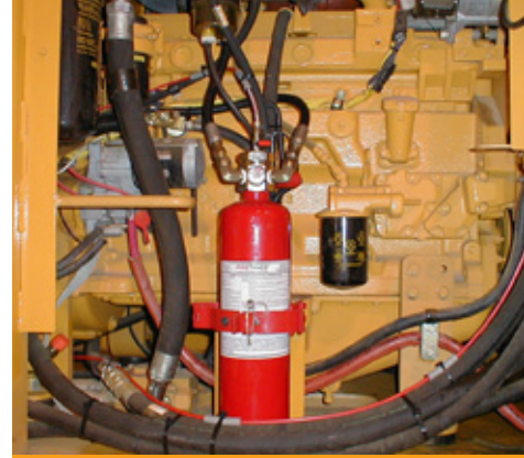
The red Firetrace cylinder can be seen here, along with the red detection tubing as it is run to the critical areas.
