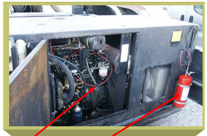
A 6KG DLP Powder System is installed to protect the generator from Fire.
